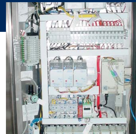
(80% less field wiring through remote I/O)
